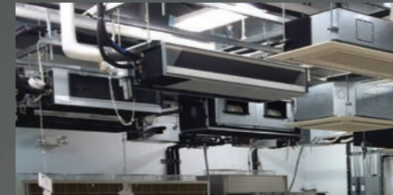
LG Air Conditioning Academy
